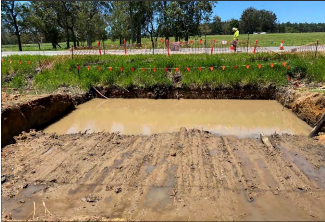
Plate 9. Thick layer of mud covering corduroy road, looking east, 28 October 2002.
