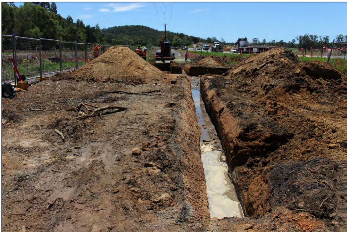
Plate 15. Strip trench showing southern extent of corduroy road indicated by yellow arrow, looking north.
