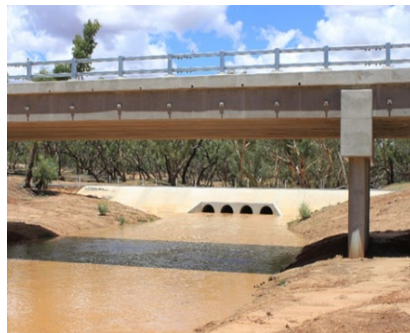
Sediment load to waterway
