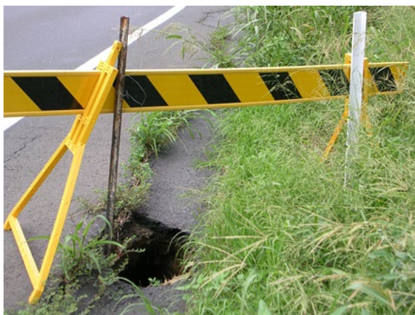
Example of tunnelling erosion in road shoulder
