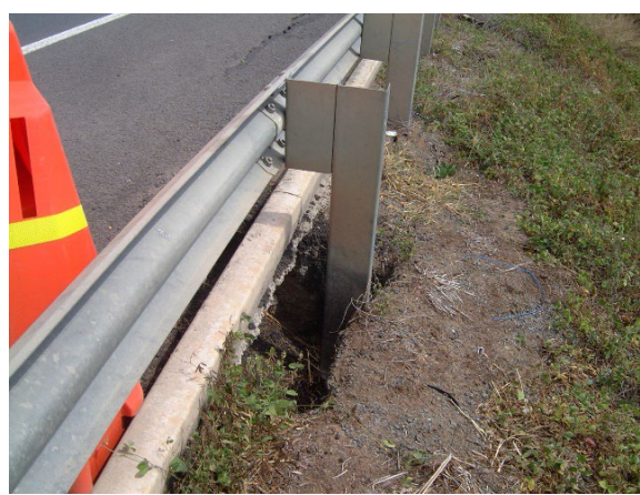
Example of void around guard rail post foundation
