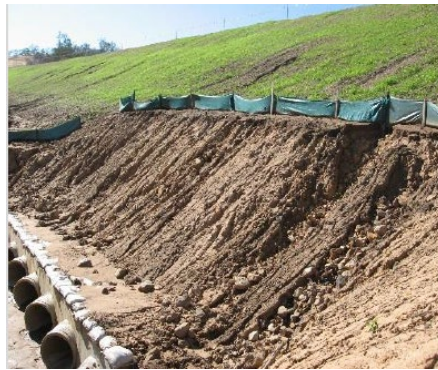
Rilled and gullied untreated embankment
