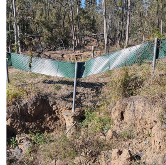
Fence footing undermined
