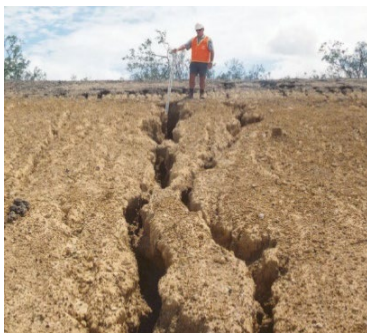
Eroded cut batter
