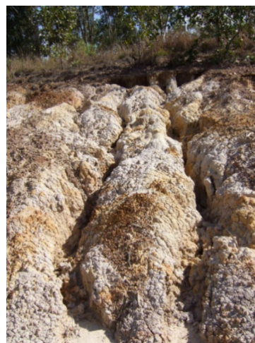
Example of rilling of cut batter
