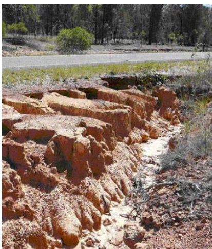
Example of gully erosion in a drainage channel
