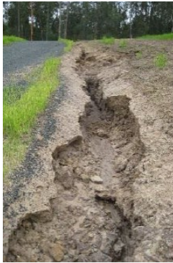
Eroded v drain
