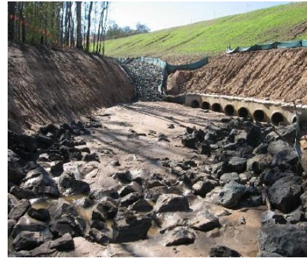
Sediment in rock-lined drain and culverts
