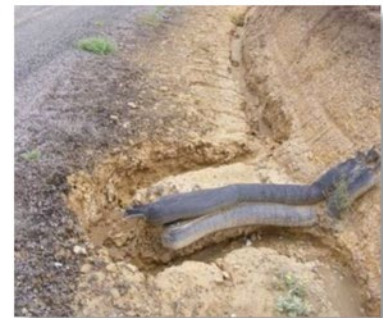
Sediment deposits and filter sock direct water around sock increasing extent of erosion.
