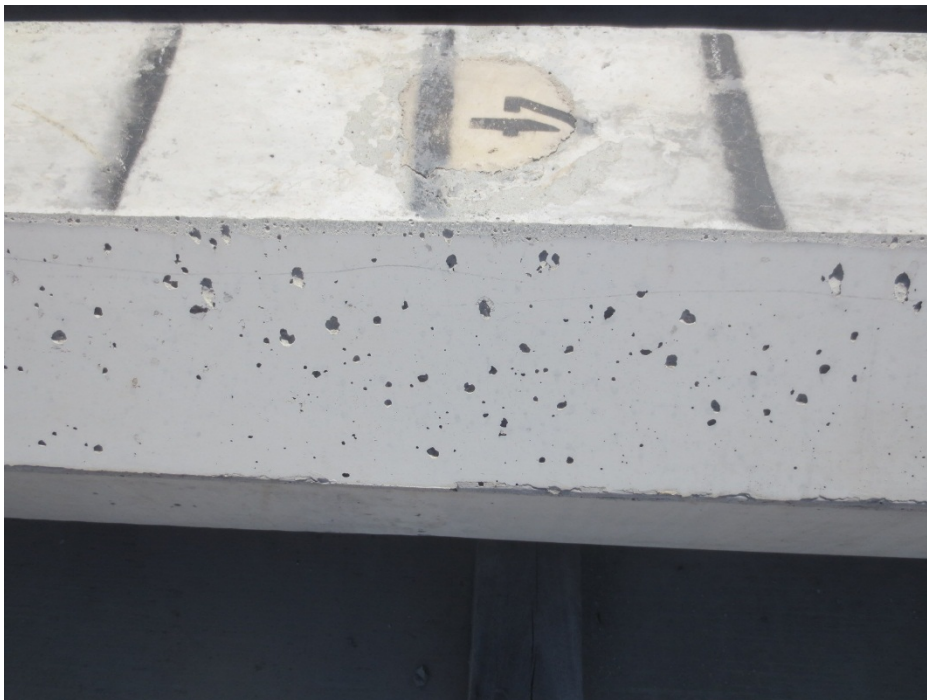
Figure 2: Unacceptable surface finish (Face D)
