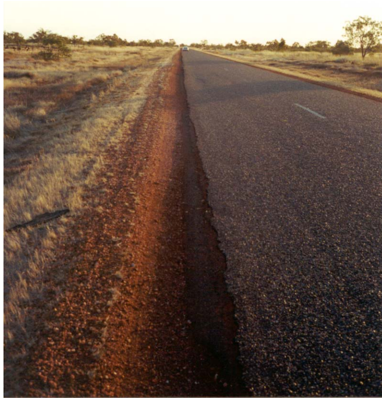
Figure 4.24 Example of inadequate single lane (5.6m) seal on a Type 2 road train route (AADT of 400 with 30% heavy vehicles)
