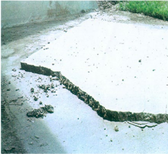
Figure 3.16(b) – Vertical displacement of apron failure
