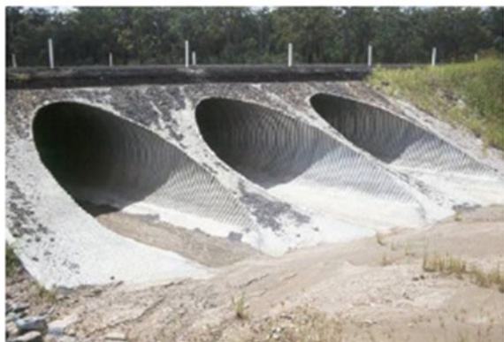
Figure 3.6.10(a) – Corrugated steel pipes
